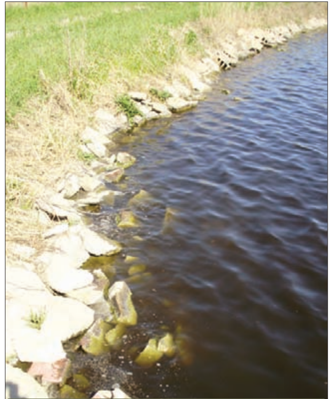
This lagoon cell is experiencing a turnover and lacks the desirable sparkling green color found in a well-operated system. Note the wastewater has a very dark brown color, some white foam developing in the stone rip-rap and very little wave action.
