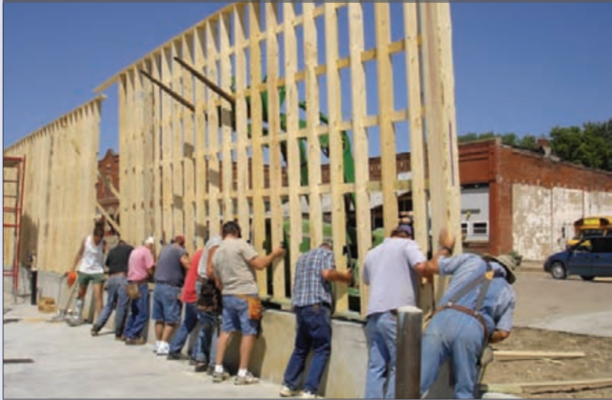
Volunteers place a section of wall for the Fire Station/Community Building in Morrill, KS. The facility covers 9,040 sq. feet.
