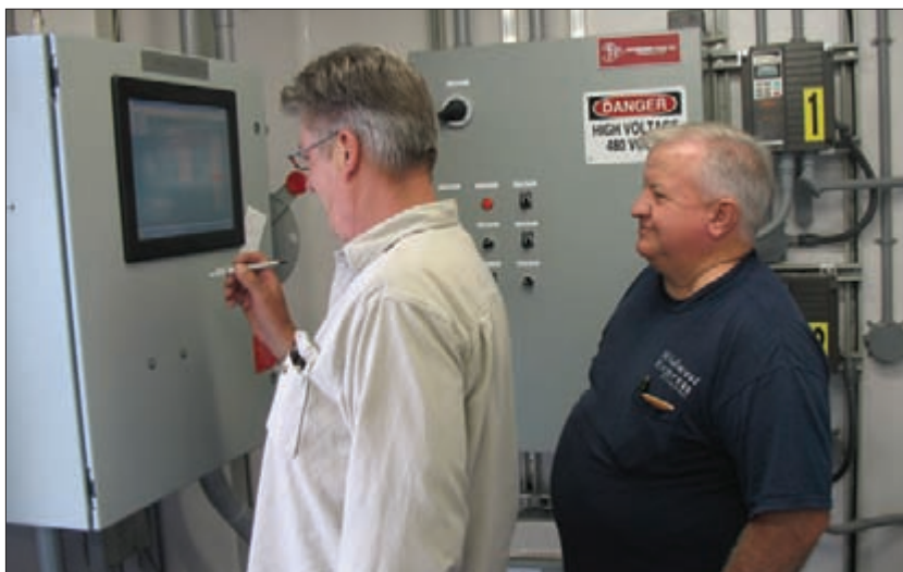
Mark Patience, operator, and Mike Ernst, board chairman, review the screen on the SCADA display inside the new pump station. The station was constructed by Engineered Systems Inc., Riverside, MO; the SCADA was installed by Micro-Comm of Olathe, KS.
