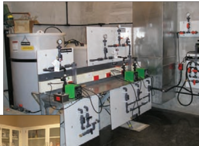
Above: The plant's chemical room administers coagulants, polymer, ammonium sulfate, and a phosphate.
