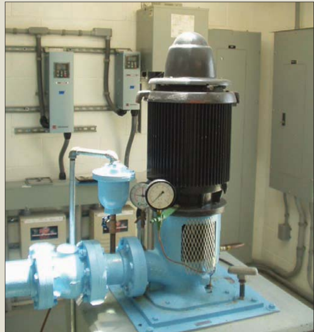
This photo shows a typical vertical turbine pump on a municipal water well in northeast Kansas. The well is adequately sealed; the vent is screened to prevent entrance of contaminants.
