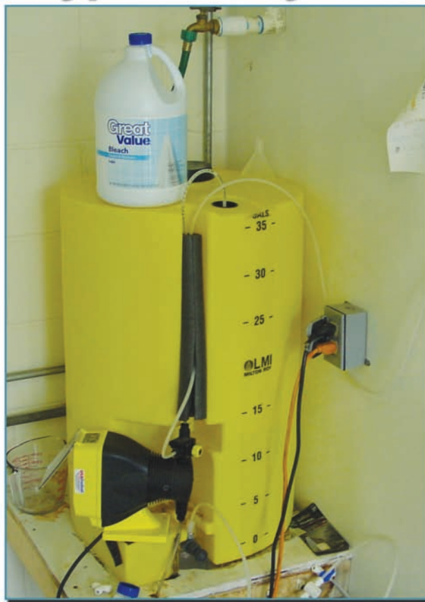
This photo shows the rechlorination system at Atchison Cons. RWD 5. The system adds six percent bleach to increase the chlorine residual. Ammonia is also added.
