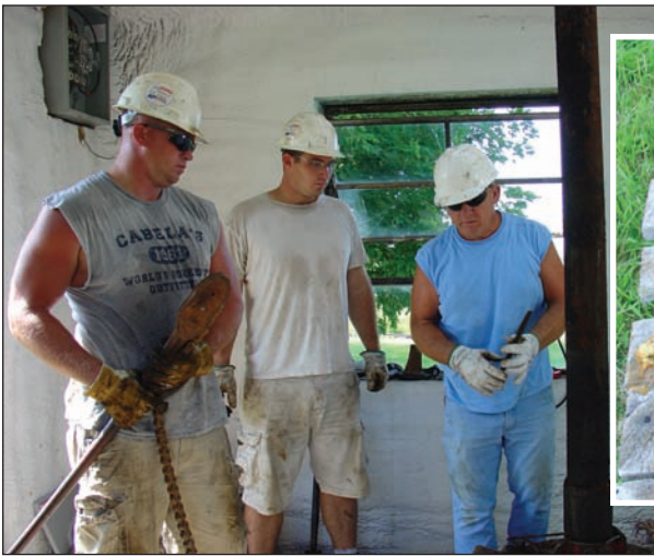
Dallas, Darren and Terry Alexander of Alexander Pump and Services, St. Marys, KS are about to remove the old column pipe and pump from the well.
