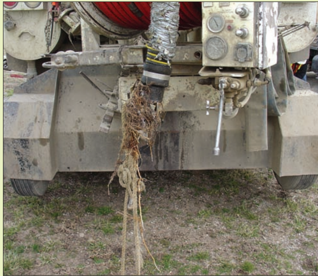
This photo shows a small bundle of tree roots that were dislodged during a cleaning project and which subsequently created a blockage in a sanitary sewer line.
