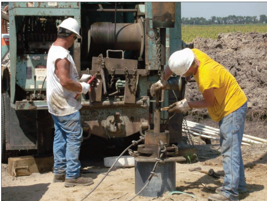
Clarke Well and Equipment of Great Bend, KS prepares to test pump the new well at Inman. The new well, connecting pipeline and new storage tank were recently completed.
