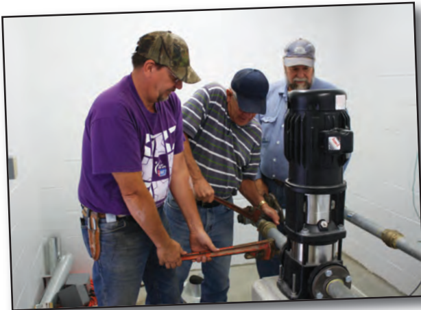
District Operator Dan Dehn is joined by Board Chairman John Davied and RWD 6 Board Member Loren Eissler in putting the final torque on the piping on the booster pump.
