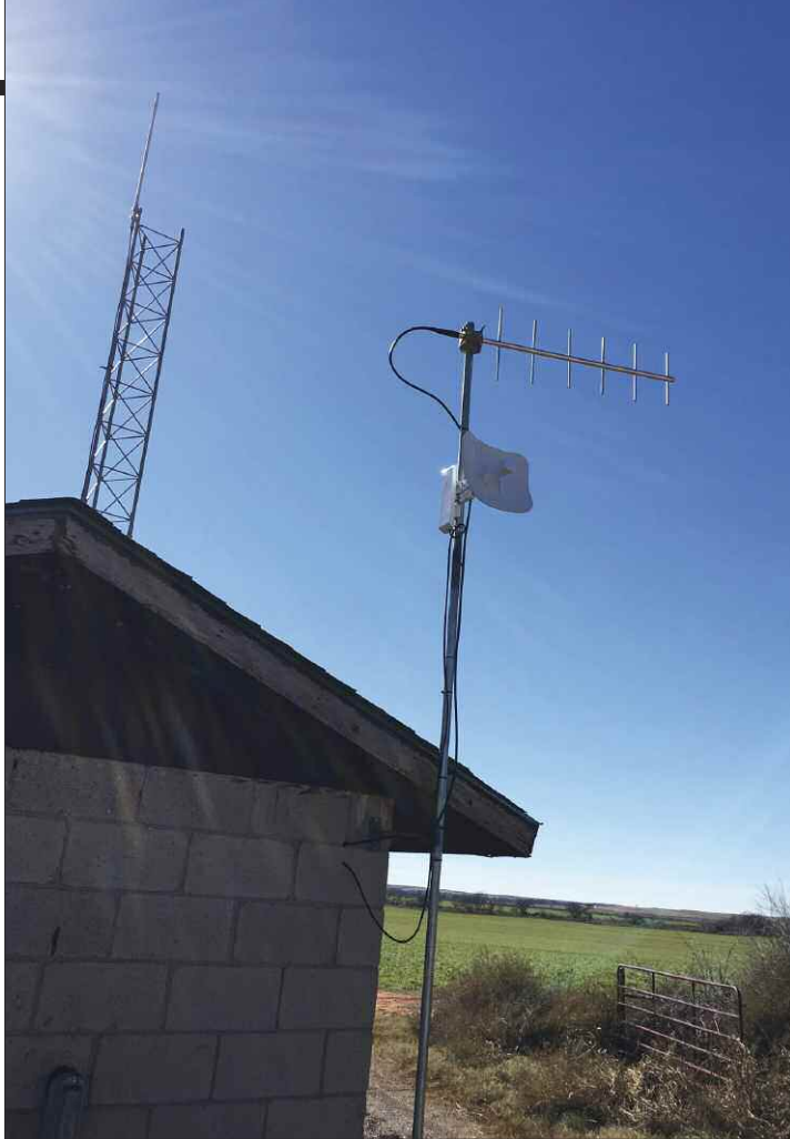
Ubiquiti LightBeam (small dish) installation at a wellhouse in Oklahoma. Photo provided by TCI.
