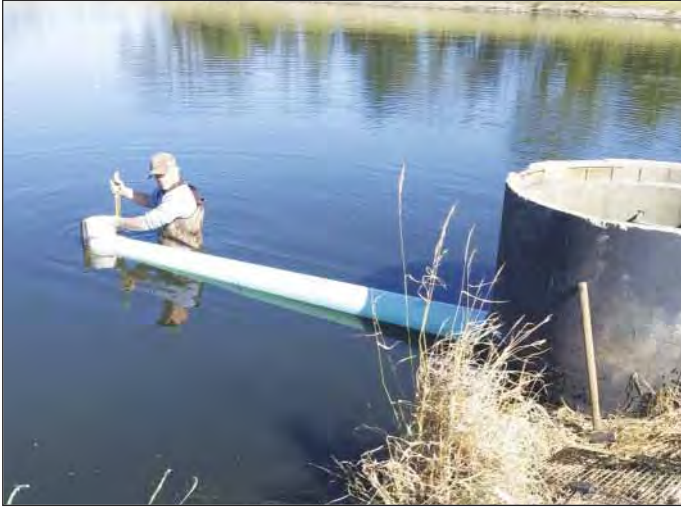
KRWA Tech Jason Solomon installs posts to support the 10-foot pipe extension.
