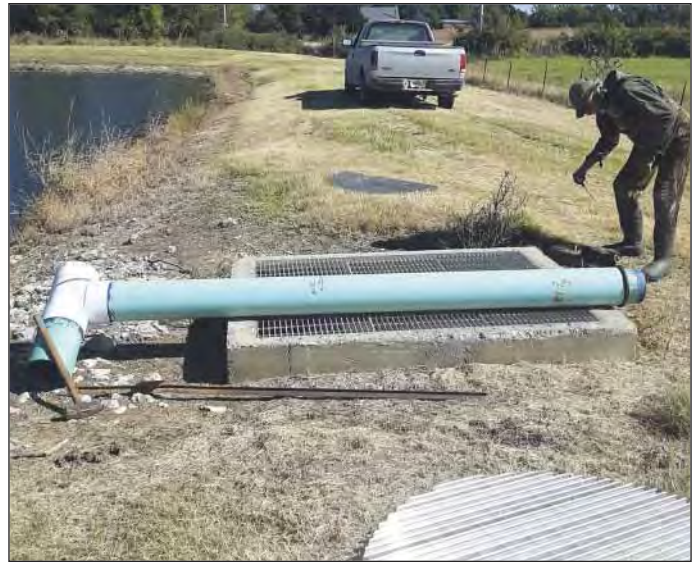
This photo shows the extension before placement in the lagoon. Notice the 90-degree tee and 20-inch downward extension that allows drawing effluent from below the water surface.
