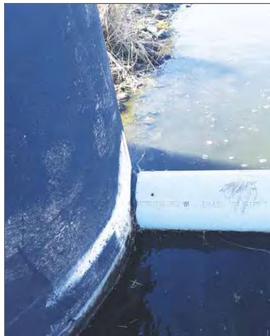
The new pipe extension connects to the existing discharge box. KRWA Tech Jason Solomon and Rex Hess, Superintendent at Mound Valley, made sure the pipe made a watertight seal with the box.
