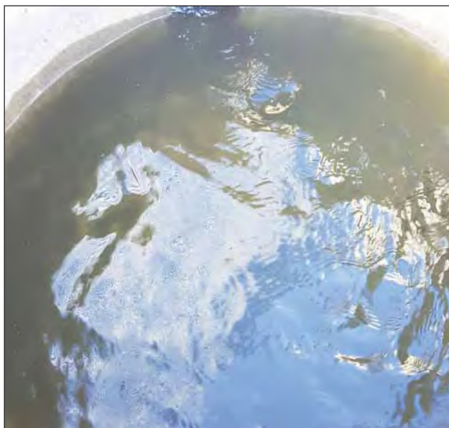
This photo shows the quality of effluent entering the discharge box before improvements. This is effluent off the surface of the lagoon. Notice the wastewater contains a lot of excessive solids, primarily due to algae.
