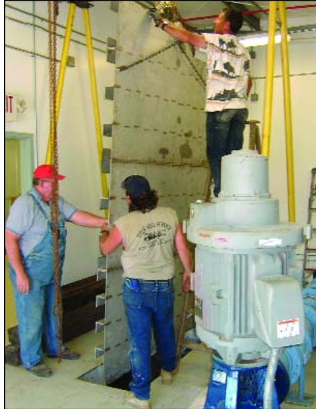
Left: Wall, hole for wall, and basin access hole in background. Above: Wall being lowered into hole. Right: Chlorine solution injection line at wall overflow.
