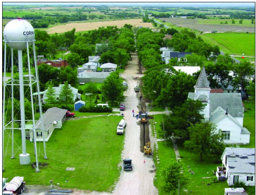
Volunteers in Corning in Nemaha County completed the installation of an entirely new water distribution system through the KAN STEP program in 2004. Kansas Commerce awarded the city a KAN STEP grant of $ 258,235 of which the city returned $ 23,846.
