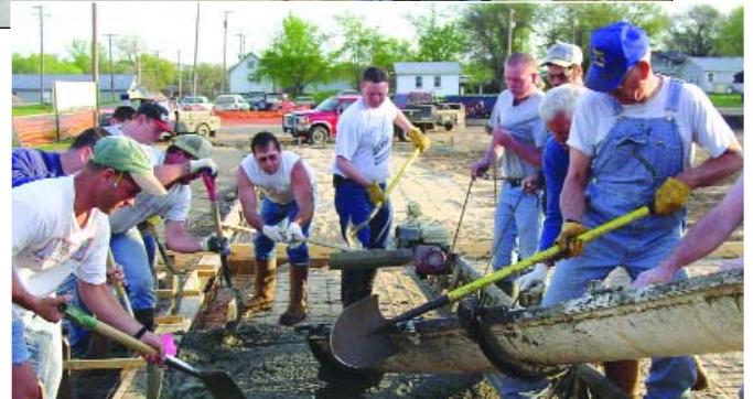
Upper photo: Volunteers in Morrill stand up a wall of their community building/fire station. The lower photo shows volunteers eagerly leveling concrete in Washington.
