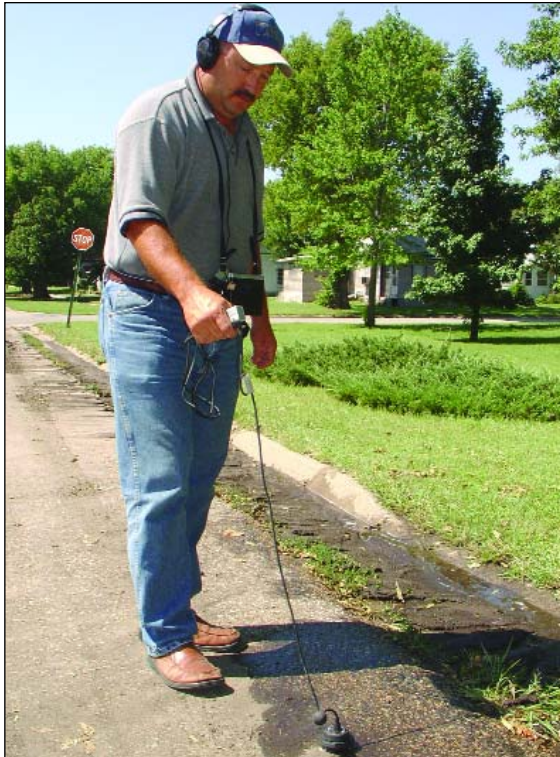
Methods for detecting leaks in water distribution systems usually involve using sonic leak detection equipment, which identifies the sound of water escaping a pipe. Pictured at the left, KRWA Tech Greg Duryea uses an ultrasonic listening device to detect sounds below ground. Other KRWA equipment includes pinpoint listening devices that make contact with valves and hydrants, and correlator devices that can listen at two points simultaneously to pinpoint the exact location of a leak, assuming the size and type of pipe are known.
