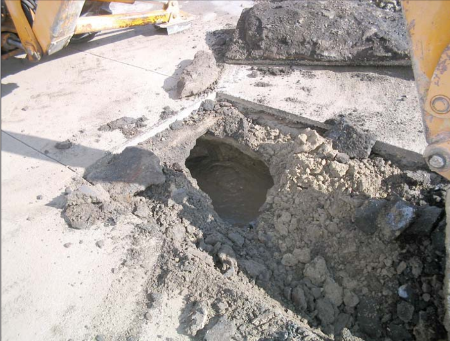
The end of the 20 plus yard-long trench is shown above. The point of the leak is seen with the water bubbling up in the hole. The crews covered the trench as they moved north so the main wouldn't freeze behind them. The frozen ground and type of soil kept the ground mic from pin pointing the leak exactly. The leak was found half way between the fire hydrant where it was first heard on the mic and the storm drain where it was heard draining into.
