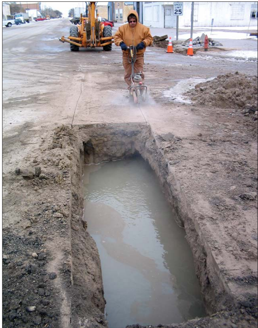
Grainfield City Council Member Joe Heier uses a concrete saw to make way for the backhoe to finish excavating the water main leak on the state highway and main street of Grainfield in January, 2008. The elusive leak caused concern with KDOT workers who saw the highway slowly develop a 20 yard patch.
