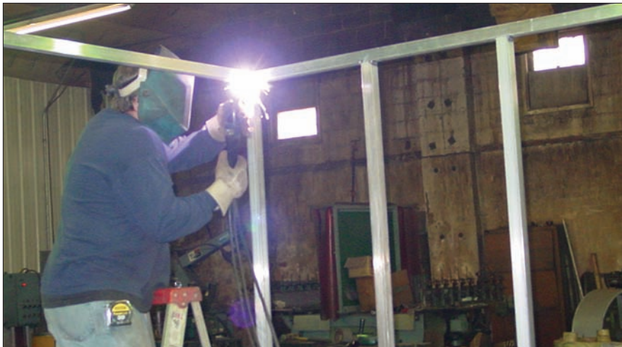
Mark Gaskell, with Horton Metal Products in Horton, KS, begins framing of the rechlorination building for Kansas Rural Water Association. The structure will be all aluminum including the frame and sheeting. Mark has also worked on other water plant projects such as basin covers. KRWA will use the station to speed correction of a system's water quality issues and also as a demonstration unit.
